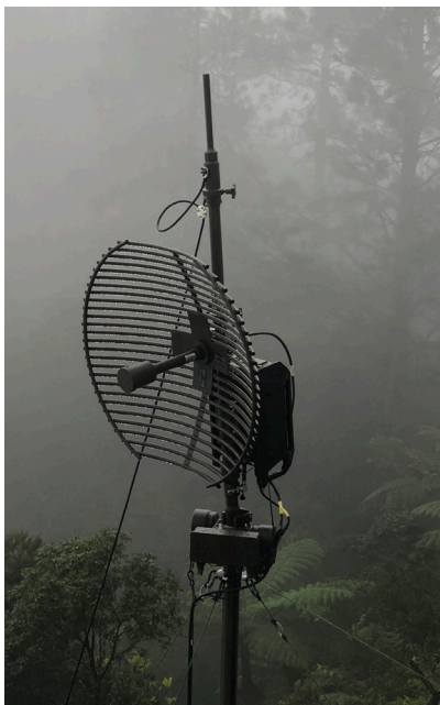
RL542A and typical antenna mounting in the rain-forest
